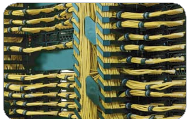
Figure 2. Elements of Cable Management with ADC KRONE Racks
