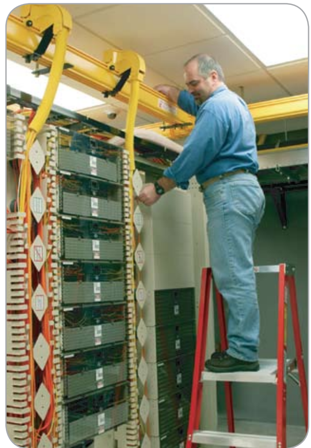
Figure 6. Elements of Cable Management with ADC KRONE Racks
