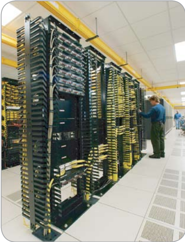
Figure 1. Equipment and Cable Racks
