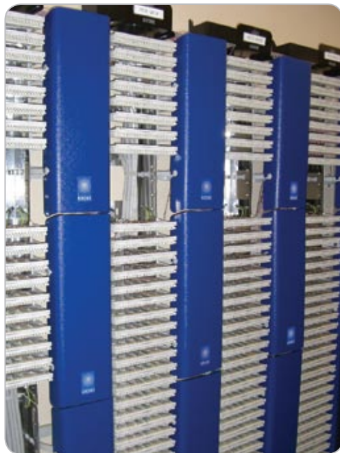
HighBand® 25 Inside The Venetian's Server Room
