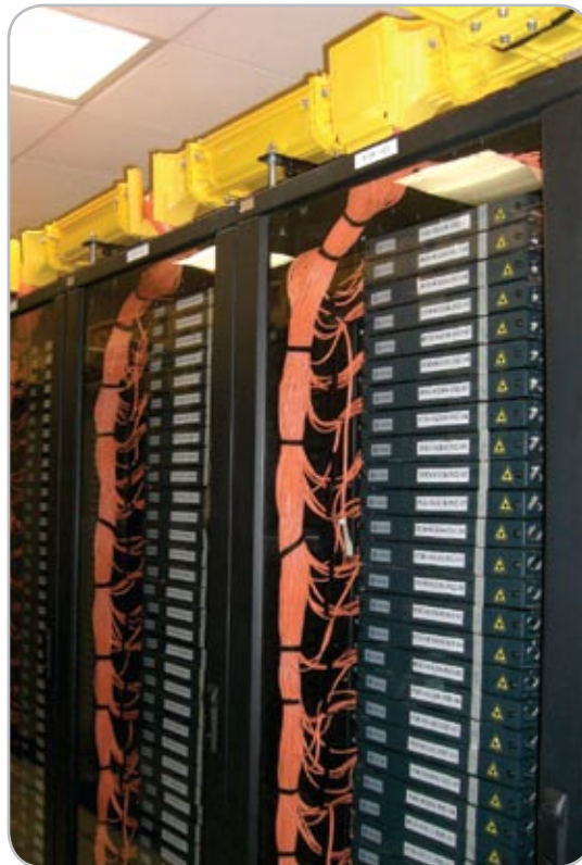
Sliding Fibre Trays with FiberGuide® Cable Management in the Server Room of The Venetian. (Macau Hotel)
